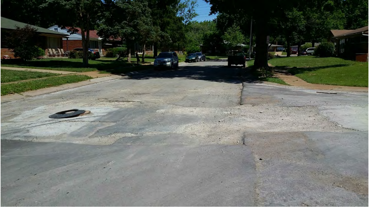
Picture 1 – 1500 block of Mendell Dr. at Milan Ave. intersection – milled road surface and protruding sewer manhole
