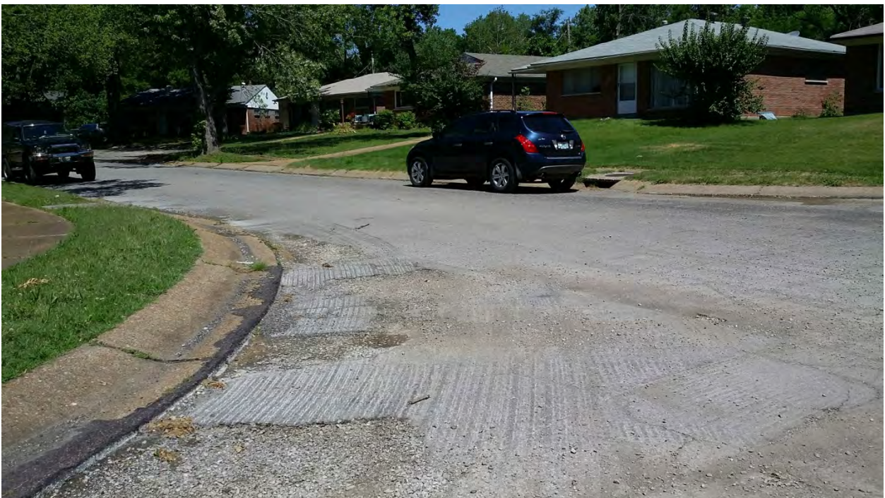
Picture 2 – 1500 block of Mendell Dr. at cul-de-sac – milled road surface
