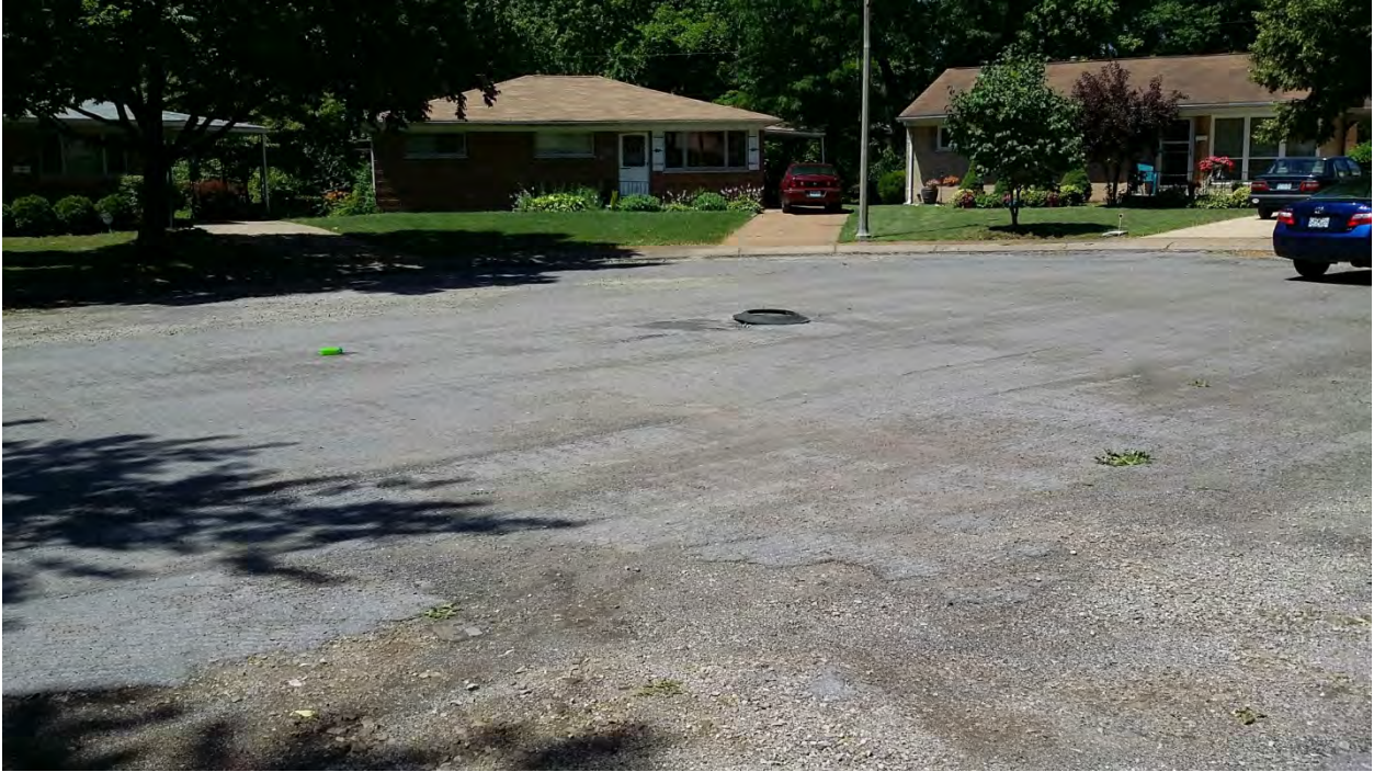
Picture 3 – 1500 block of Mendell Dr. at northern end – milled road surface and protruding sewer manhole
