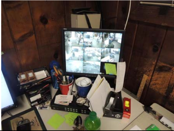
PHOTO #31: Security system
