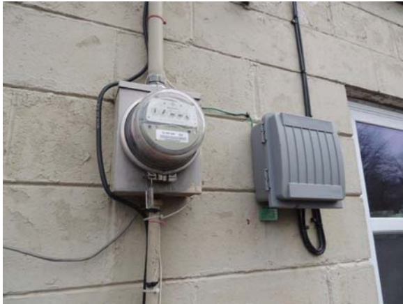
PHOTO #7: Electrical meter
