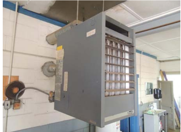
PHOTO #10: Gas fired unit heater
