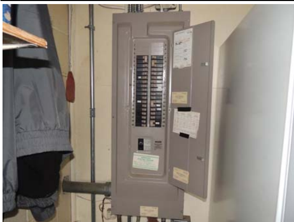
PHOTO #29: Incoming electric service
