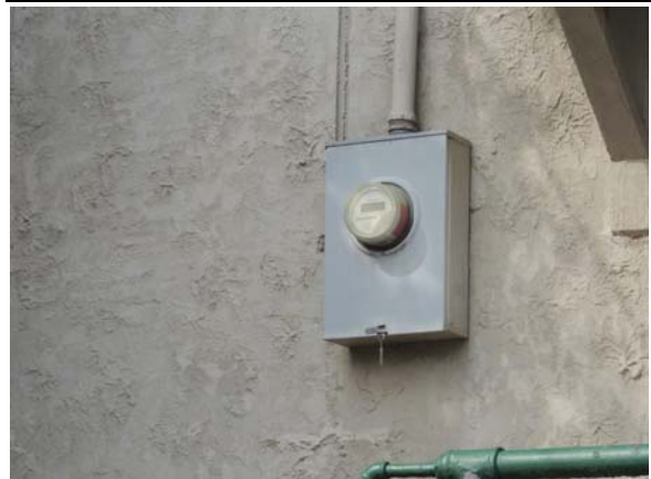
PHOTO #22: Electric meter
