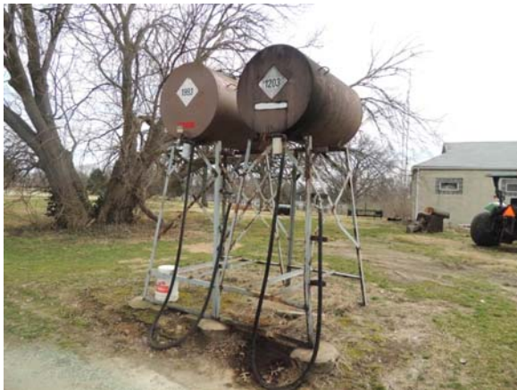
PHOTO #29: Fuel tanks
