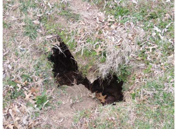
PHOTO #8: Sinkhole at rear of property suspected to be associated with the septic system
