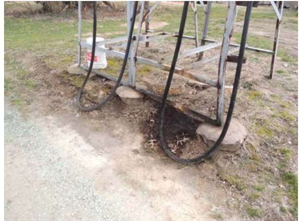
PHOTO #30: Ongoing contamination from fuel tanks
