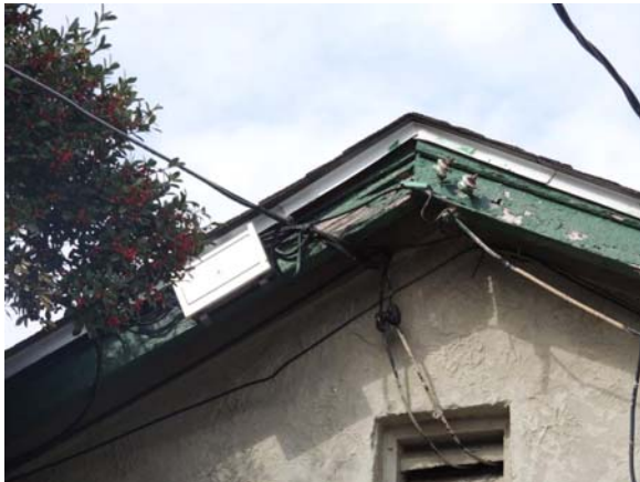
PHOTO #13: Deteriorated exterior trim
