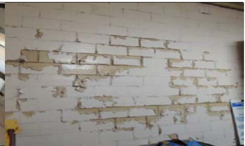
Peeling wall paint
