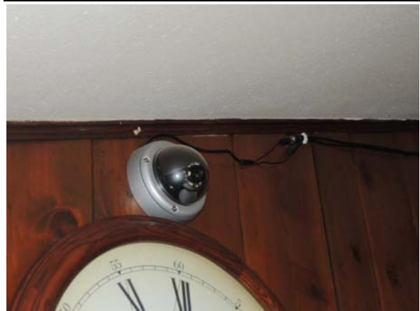
PHOTO #30: Security system
