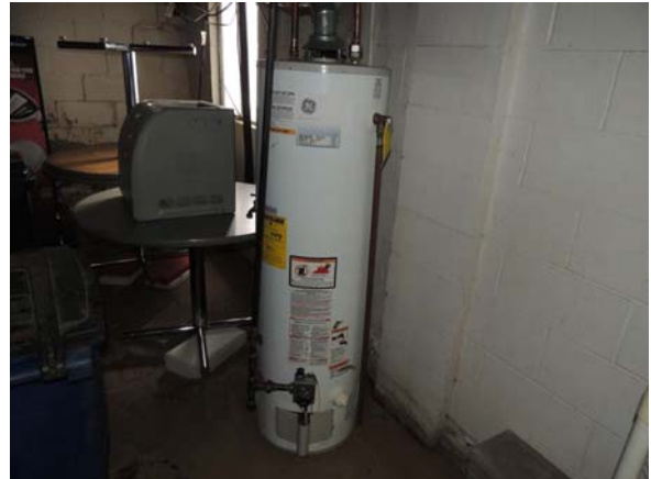
PHOTO #28: Gas-fired water heater
