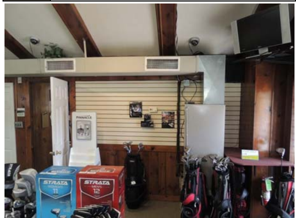
PHOTO #24: Exposed ductwork
