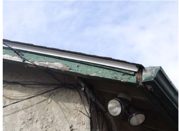
PHOTO #14: Deteriorated exterior trim
