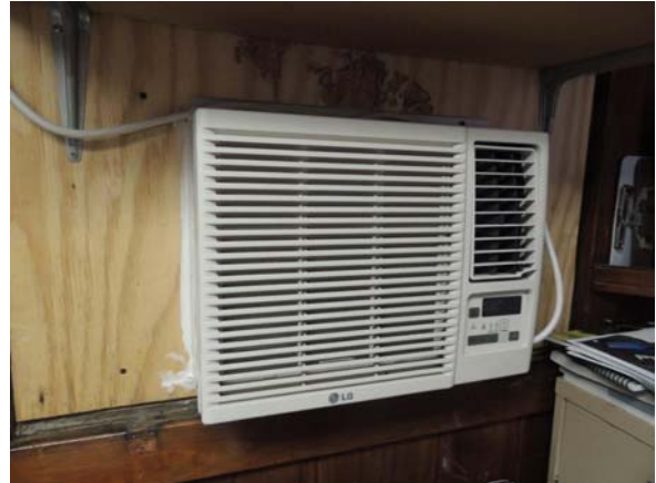
PHOTO #26: Window air conditioner
