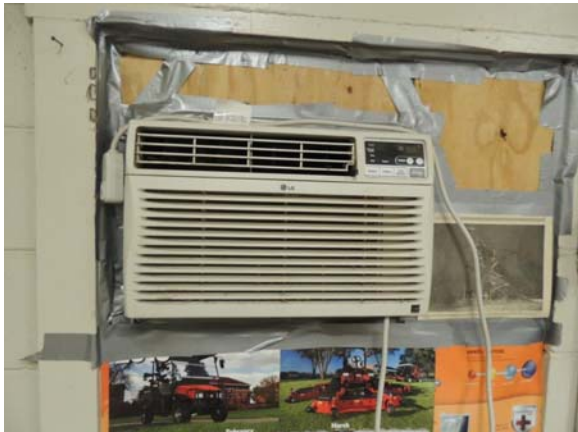
PHOTO #9: Window air conditioner
