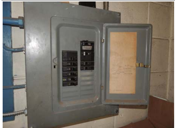
PHOTO #12: Incoming electrical service
