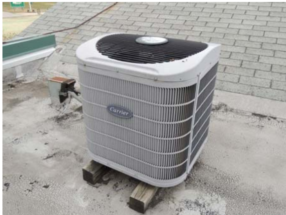
PHOTO #19: Roof mounted condensing unit
