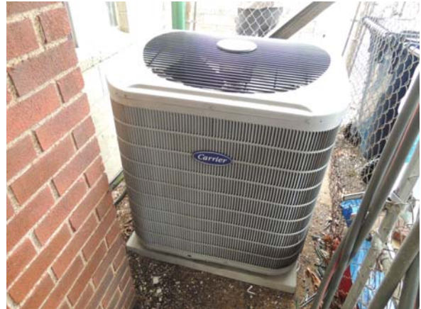
PHOTO #20: Grade mounted condensing unit
