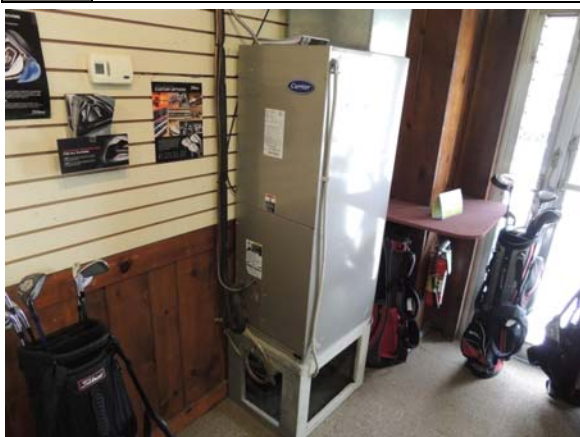
PHOTO #23: Air handling unit
