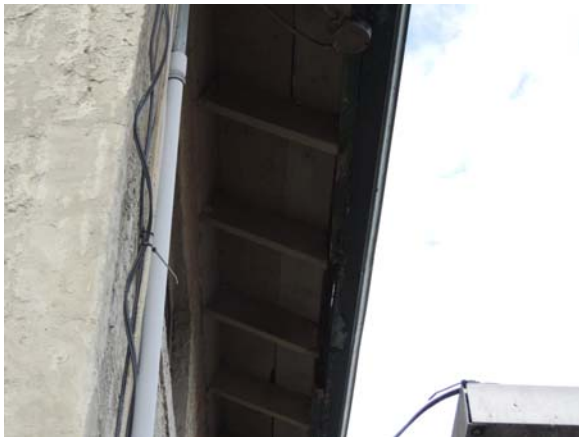
PHOTO #15: Deteriorated exterior soffit
