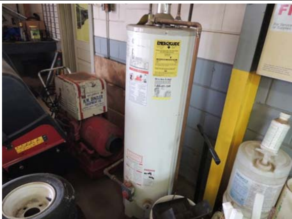
PHOTO #11: Gas-fired water heater
