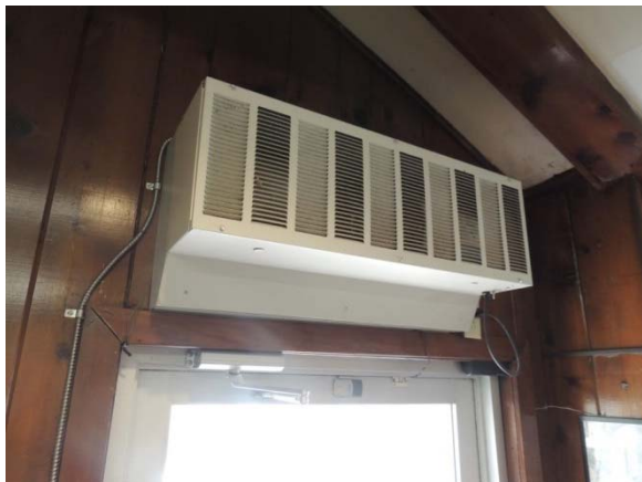
PHOTO #27: Air curtain
