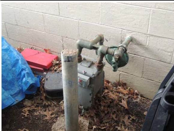
PHOTO #21: Gas meter
