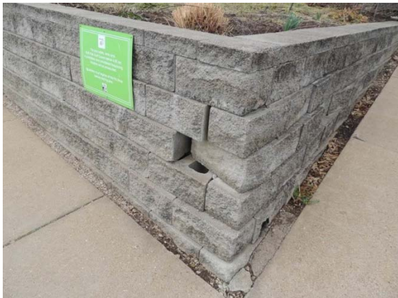
PHOTO #17: Damaged retaining wall
