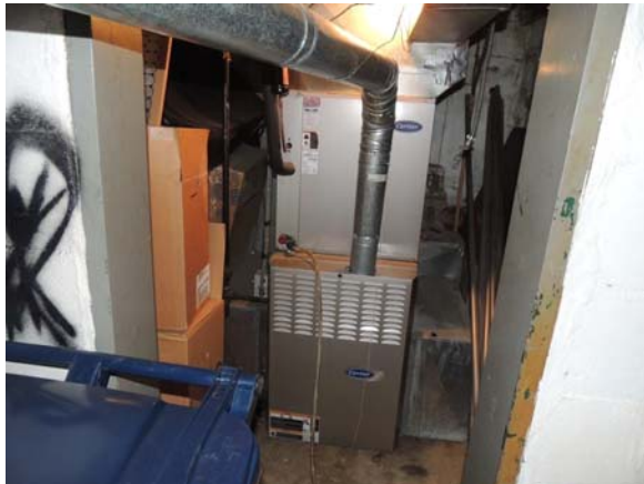
PHOTO #25: Gas fired furnace
