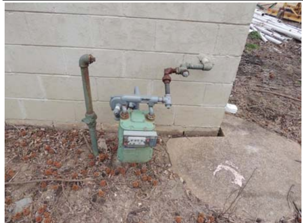
PHOTO #6: Gas meter
