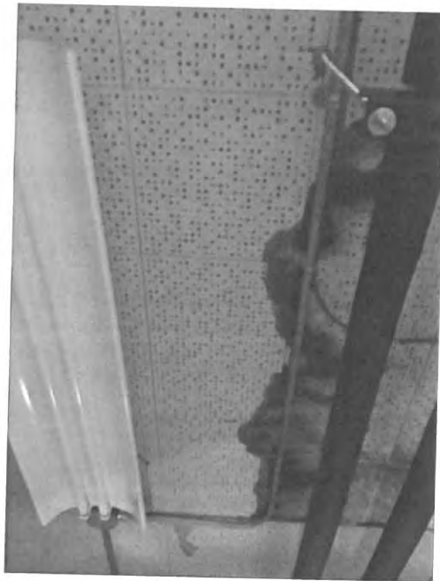
Interior water damage due to deferred maintenance of air conditioner units throughout.
