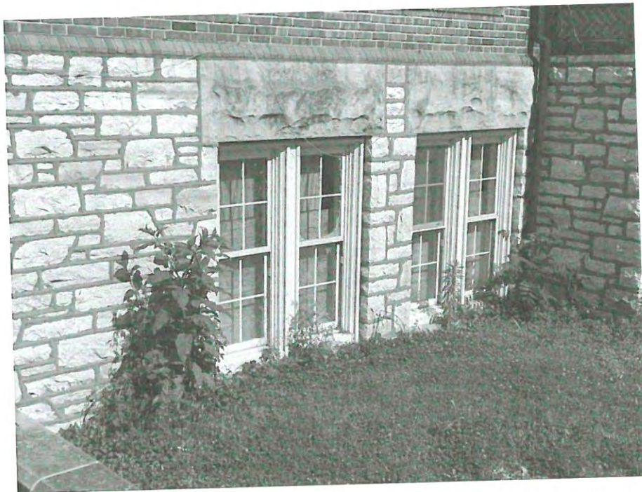
Poor drainage and window placement, which resulted in water intrusion into the interior building.
