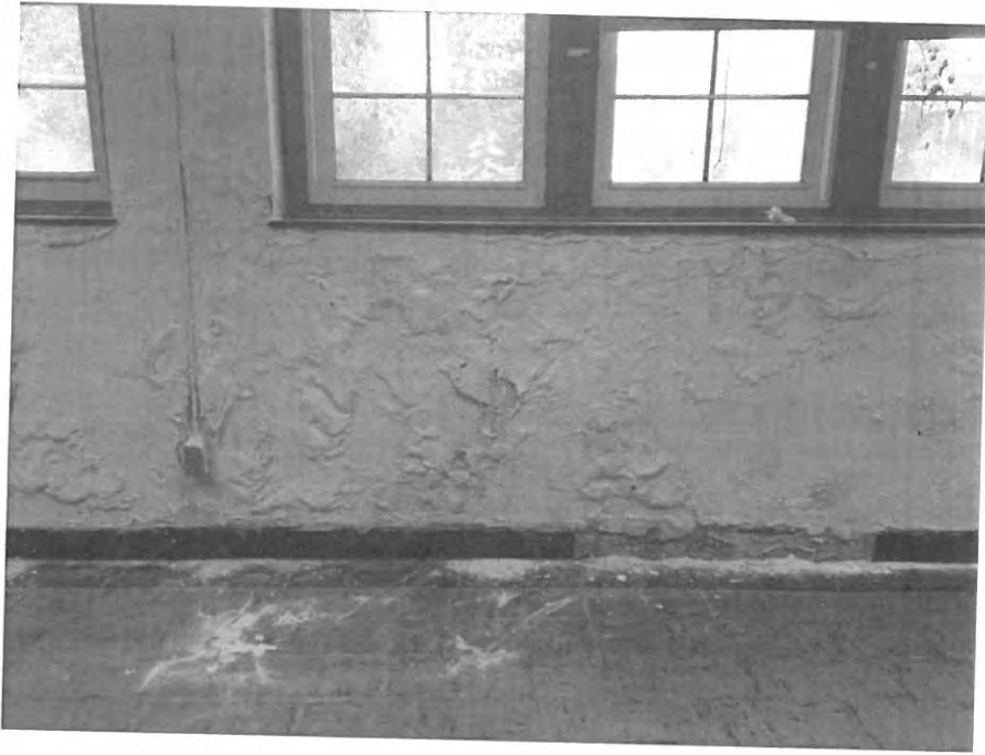
Water damage and peeling paint in classroom on second floor.
