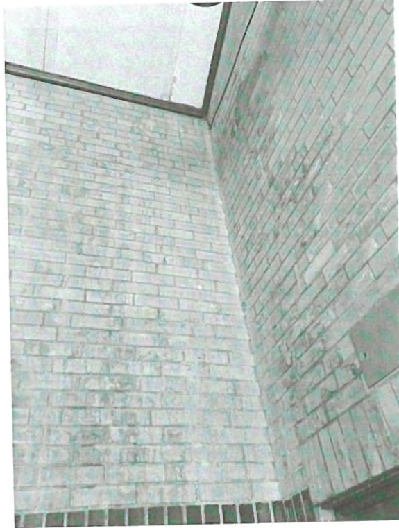
Evidence of water intrusion in the gymnasium.
