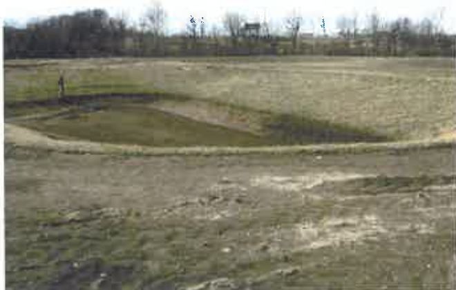
Surface Sand Filter Clogged with Construction Site Sediment, Berkeley, MO
