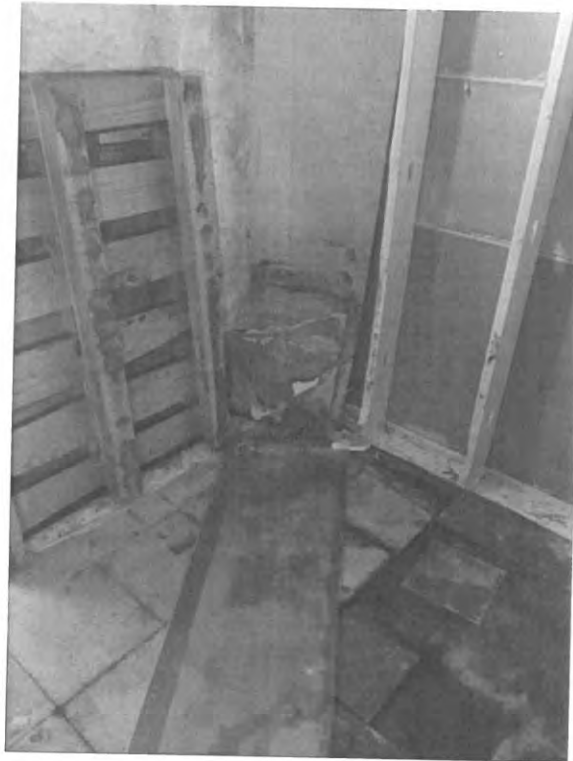
Exterior wall exhibiting water damage and mold on first floor.
