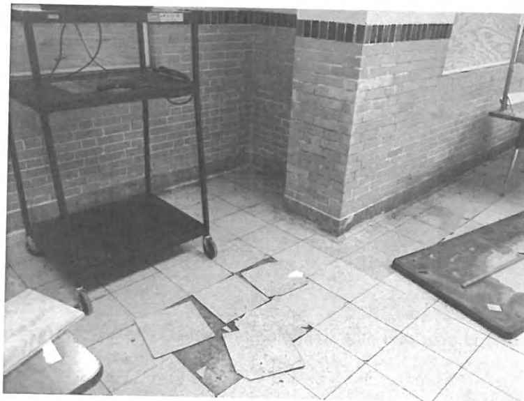
Water damage, debris, and mastic tile common throughout.
