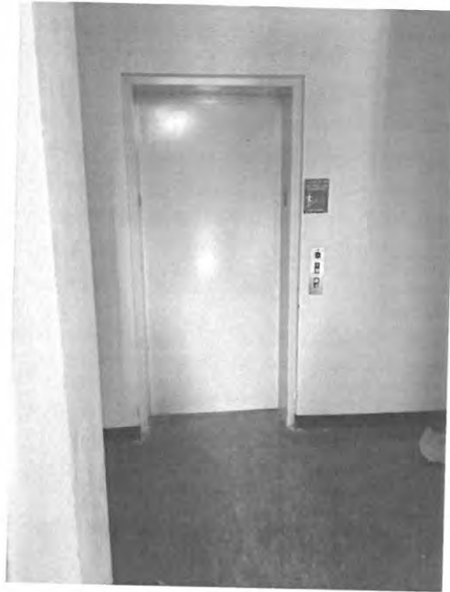
Non-functional elevator located near steps without ADA compliant ramp located on the first floor.
