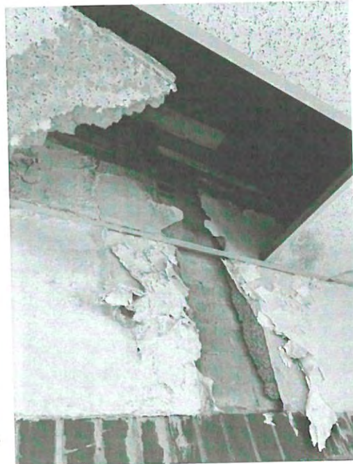
Significant water damage to classroom on first floor.
