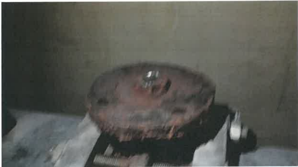
VALVE HOUSING WITH SHAFT STEM MISSING
