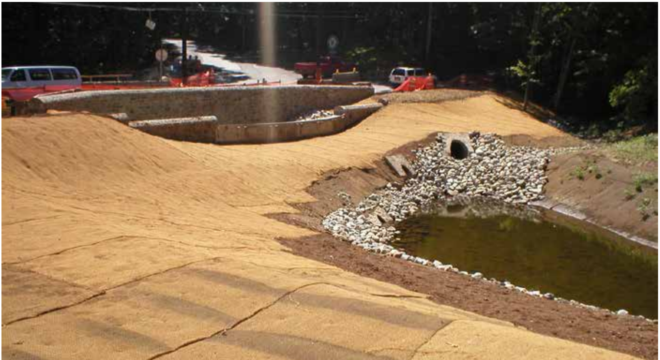
Erosion and sediment control measures in place during construction of a BMP in the Staten Island Bluebelt, NY
