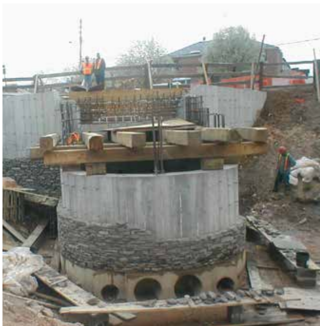
Structural control of stormwater flow in the Staten Island Bluebelt in New York City, NY
