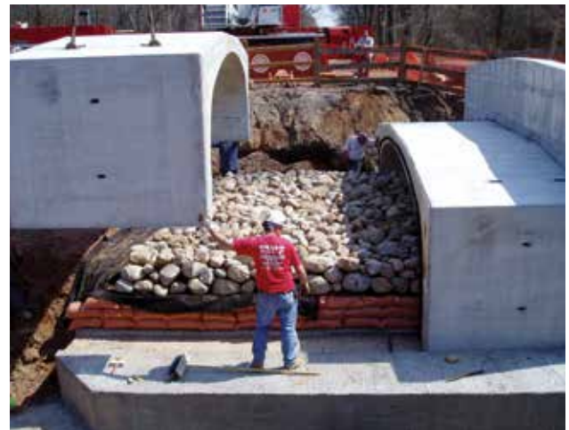
Rough bottom culverts were used to maintain fish passage.
