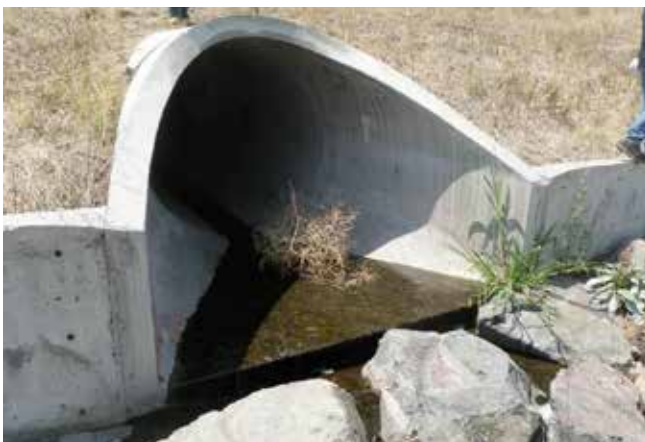
Stormwater outfall with dry weather discharge actively flowing in Aurora, CO
