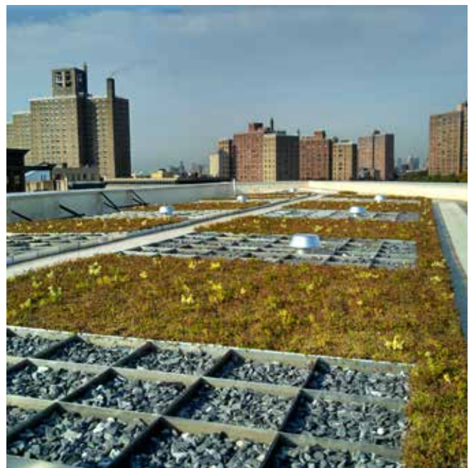
Osborne green and blue roof in New York City, NY
