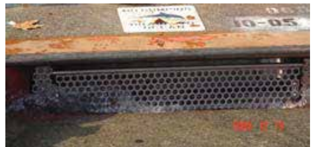
Flow-activated catch basin cover in Los Angeles, CA
