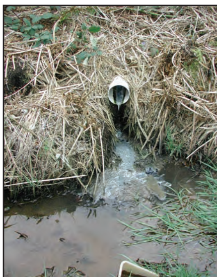
Figure 2: Direct Discharge from a Straight Pipe
