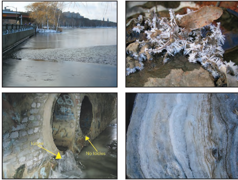
Figure 41: Cold climate indicators of illicit discharges
