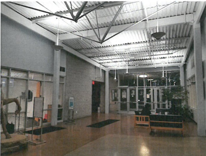
Lobby LED Lighting
