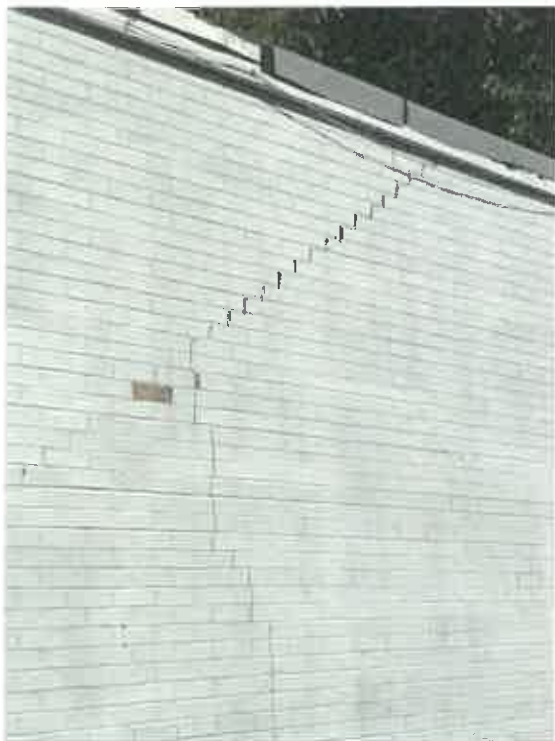
Step-cracking in this commercial building is an indication of deterioration and a structural deficiency that requires repair.
