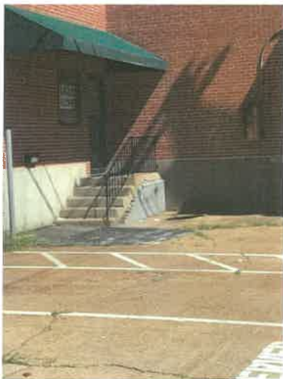
Another view of the stairwell shown in the photo above. Notice that the stairwell appears to be supported by stacks of cinder blocks.
