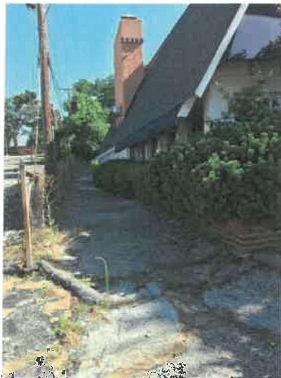
Deteriorated pavement and fencing along the side of a business on Olive.
