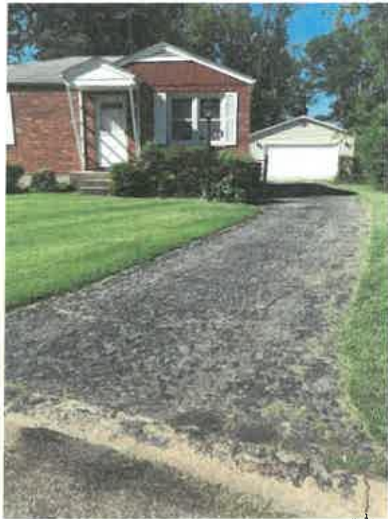
Deteriorated residential driveway in need of replacement.
