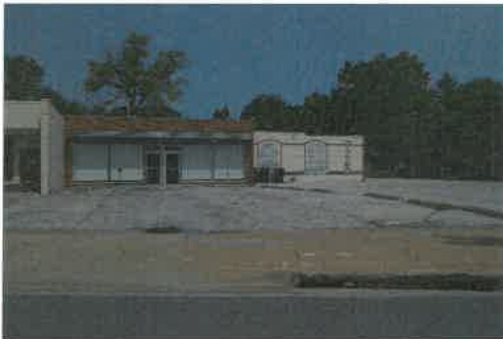
A vacant, deteriorated commercial building along Olive.
