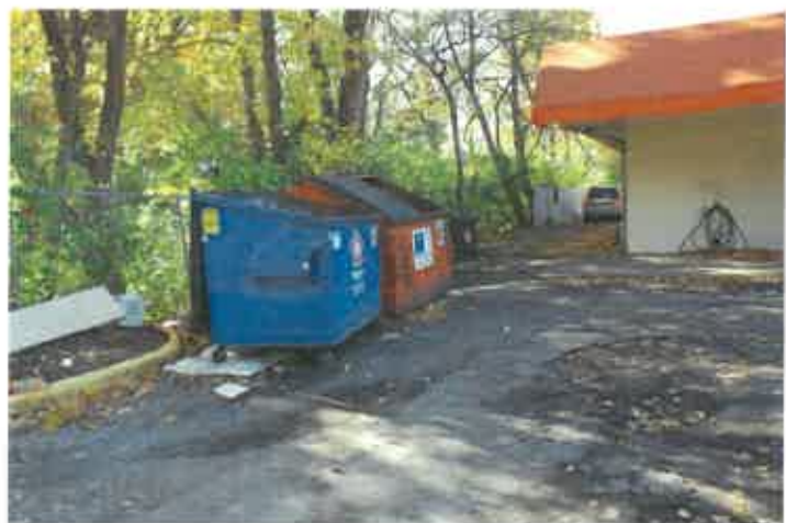
Deteriorated paved surfaces.
