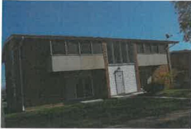
Deteriorated multi-family building.
