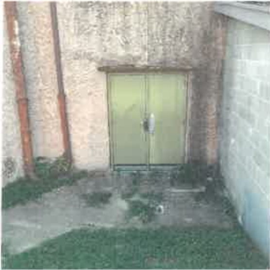
Deteriorated gutter downspouts, door, and pavement. Water damage is evident on exterior of the building.
