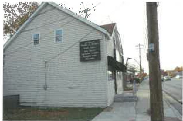
This commercial building shows signs of deterioration affecting siding material and foundation.
