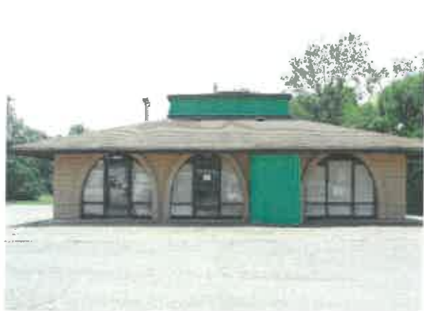
Deteriorated, vacant commercial restaurant building.
