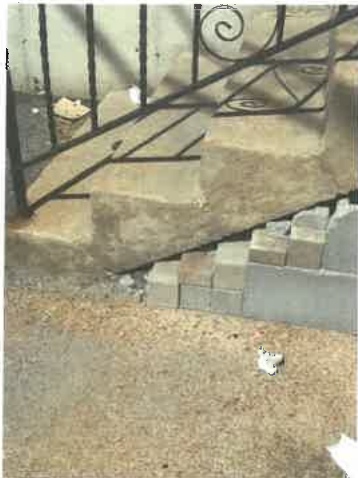
Deteriorated stairwell at rear of a commercial building.
