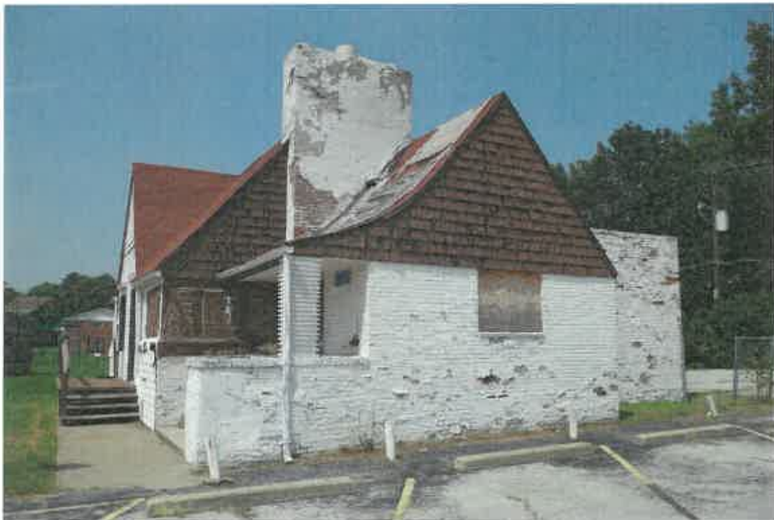
A deteriorated, dilapidated, abandoned building that evidently began its life as a residence, was converted for commercial use, and then abandoned. It suffers from significant deterioration to primary and secondary building components.
