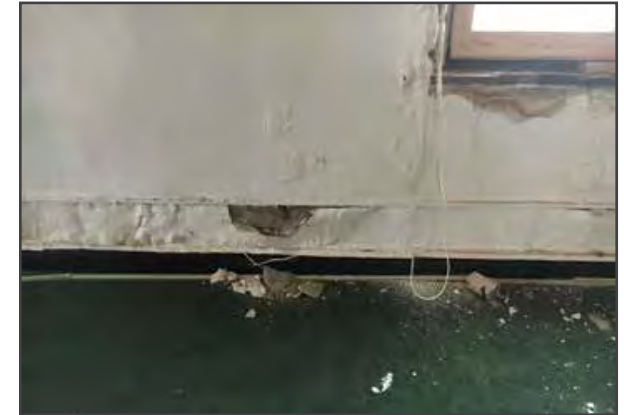
09.02 GYPSUM PLASTERING Spalling
