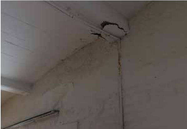
03.00 CONCRETE Spalled Beam
