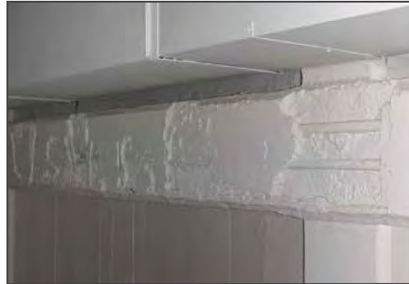
03.03 SPALLED CONCRETE COVER AT ROOF BEAM Spalling
