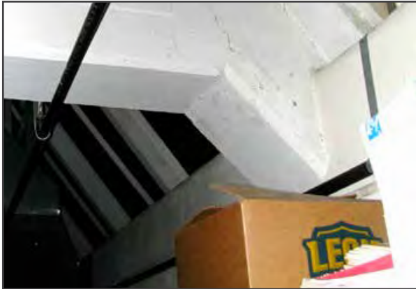
03.03 CRACKS IN MAIN ROOF BEAMS AT MONITOR Cracking
