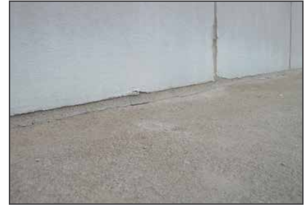
04.03 CRACKED RE-POINTING MORTAR & SPALLING PAINT AT TERRACOTTA
