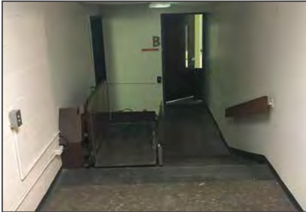
14.01 ELEVATOR Lift General Condition
