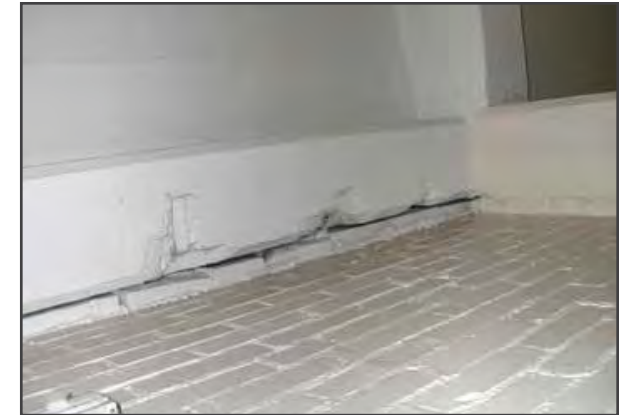
04.20 NORTH WALL GAP AT FLOOR BEAM
