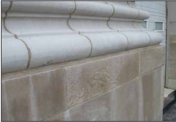
04.03 SPALLING PAINT ON TERRACOTTA
