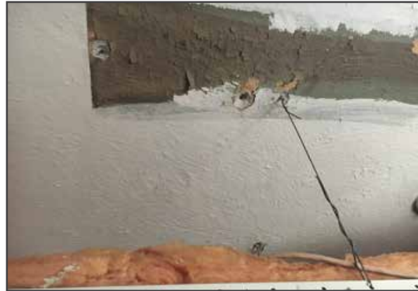
09.01 PAINT Peeling Paint
