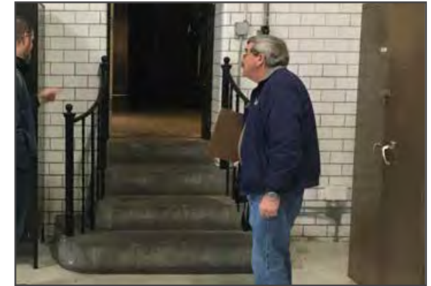
05.03 DECORATIVE METAL RAILINGS Non-Code Compliant
