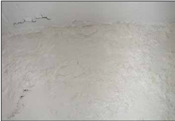
04.03 BUBBLED PAINT FROM MOISTURE INFILTRATION
