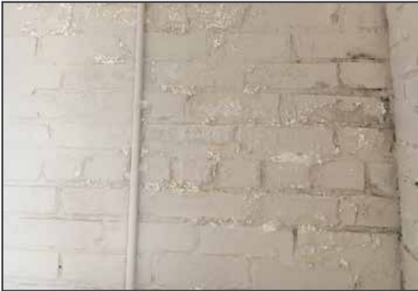
09.01 PAINT Exterior Wall Efflorescence
