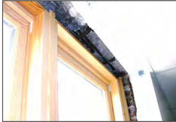
03.03 RUSTED REBAR AT WINDOW LINTELS Freeze-Thaw Damage
