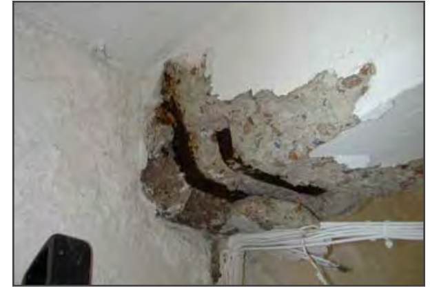
03.03 SPALLED CONCRETE AT ROOF BEAM Overload Condition
