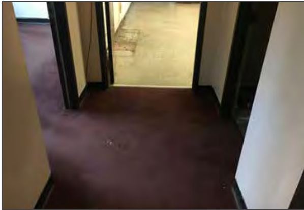
09.11 SHEET CARPETING Stained/Crushed Pile
