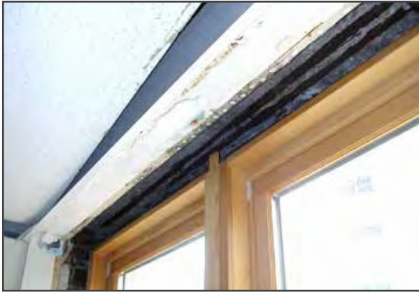
03.03 RUSTED REBAR AT WINDOW LINTELS Natural Seams
