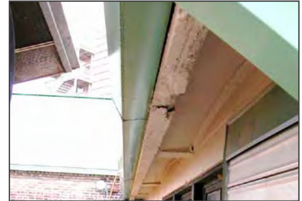
03.03 SPALLED CONCRETE COVER AT MONITOR ROOF Spalling
