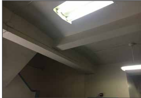
26.01 INTERIOR LIGHTING General Condition
