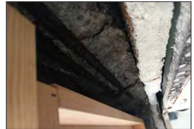
03.00 CONCRETE Deteriorated Lintel
