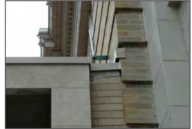
04.03 LOOSE BRICK AT GARAGE
