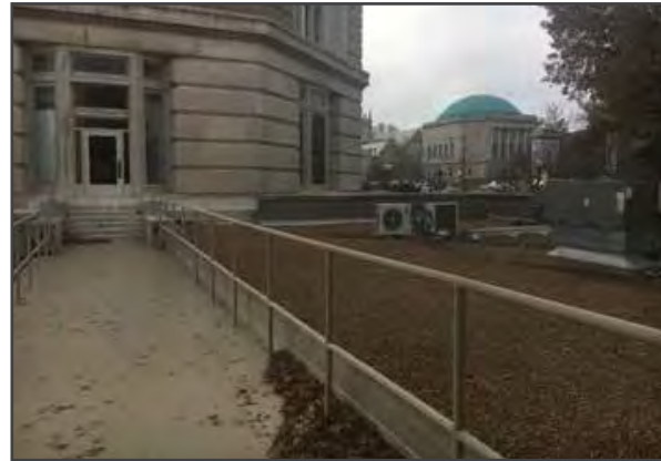
05.03 DECORATIVE METAL RAILINGS Inconsistent styling
