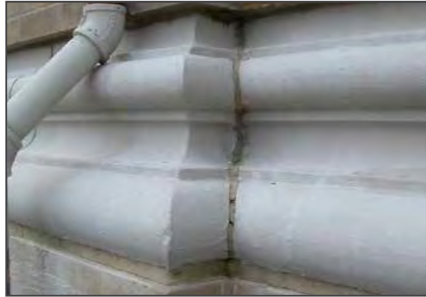
04.03 SPALLING RE-POINTING MORTAR
