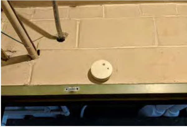
28.01 ELECTRONIC SAFETY & SECURITY Fire Alarms
