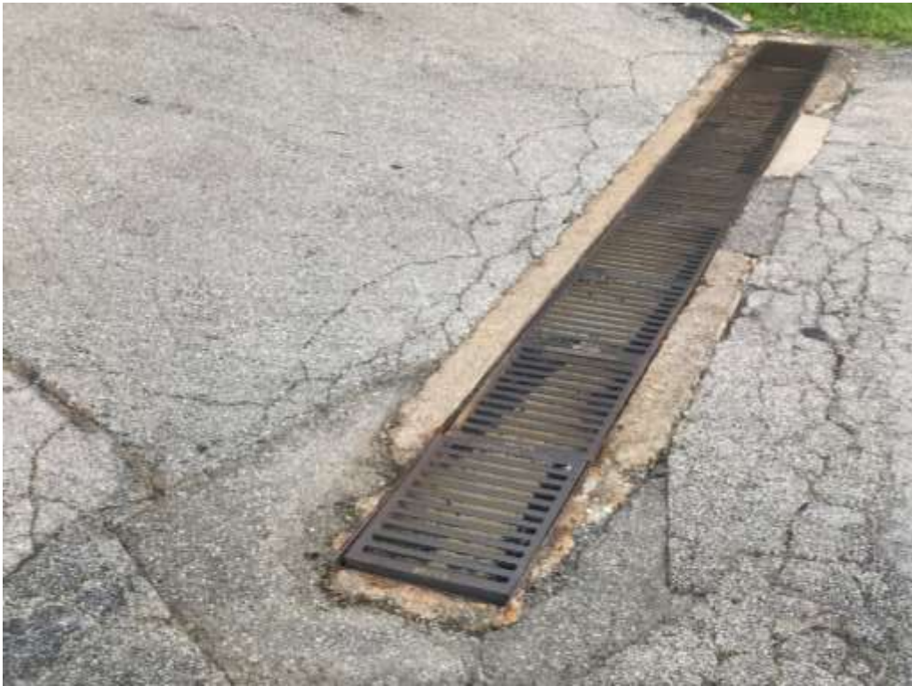
Deteriorated storm water inlet and parking surface area
