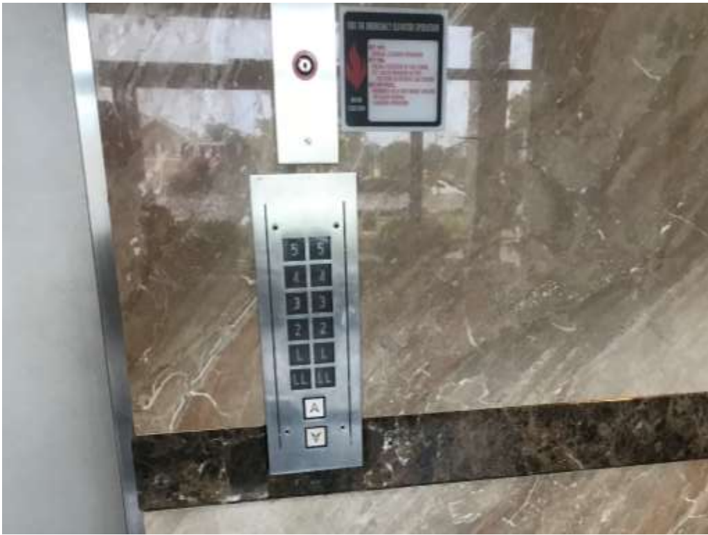
Inaccessible elevator hallway call buttons
