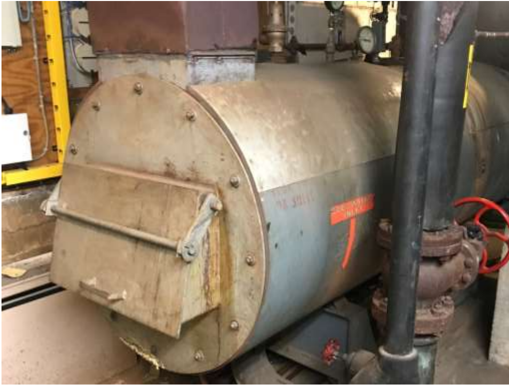
Original boiler for 8420 Building heating plant
