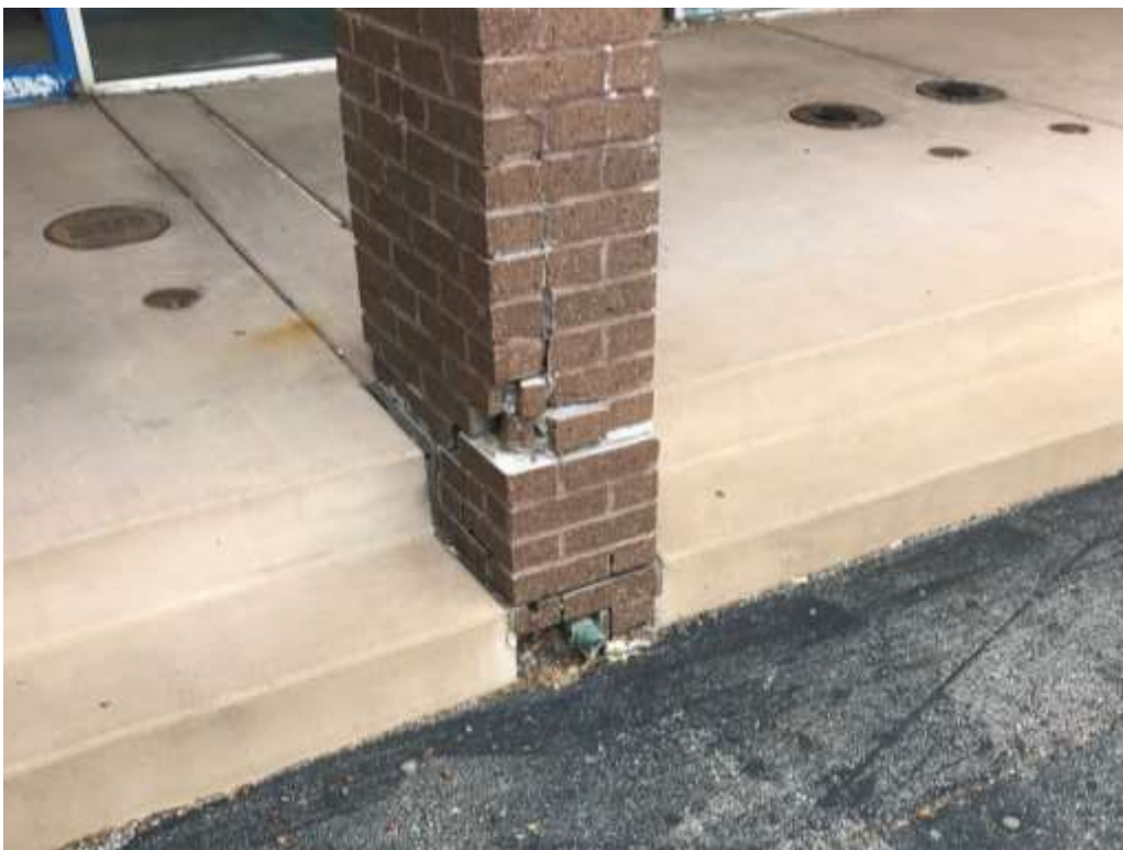
Deteriorated brick column at main entry of 8420 Building
