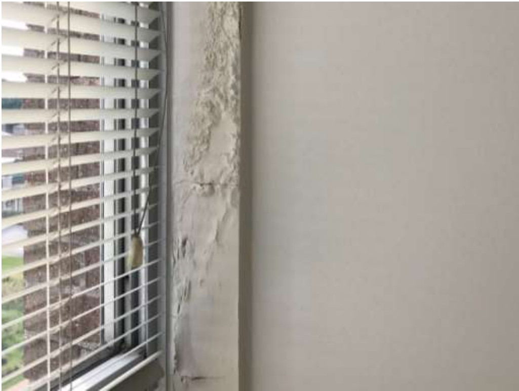
Indication of water penetration fifth floor west office space of 8420 Building
