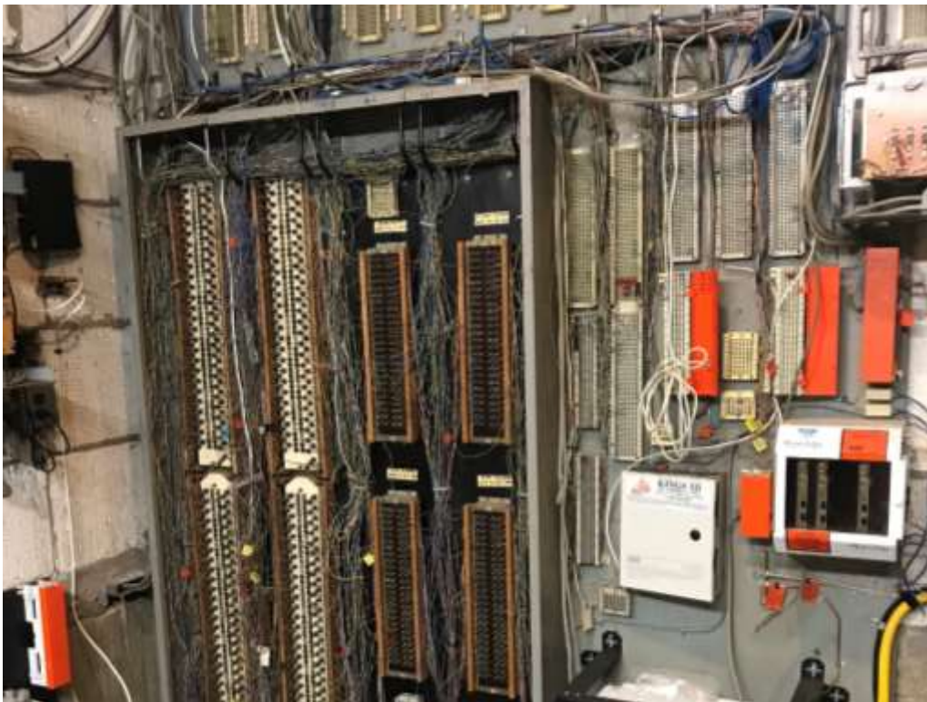
Obsolete communications wiring in utility area of 8420 Building
