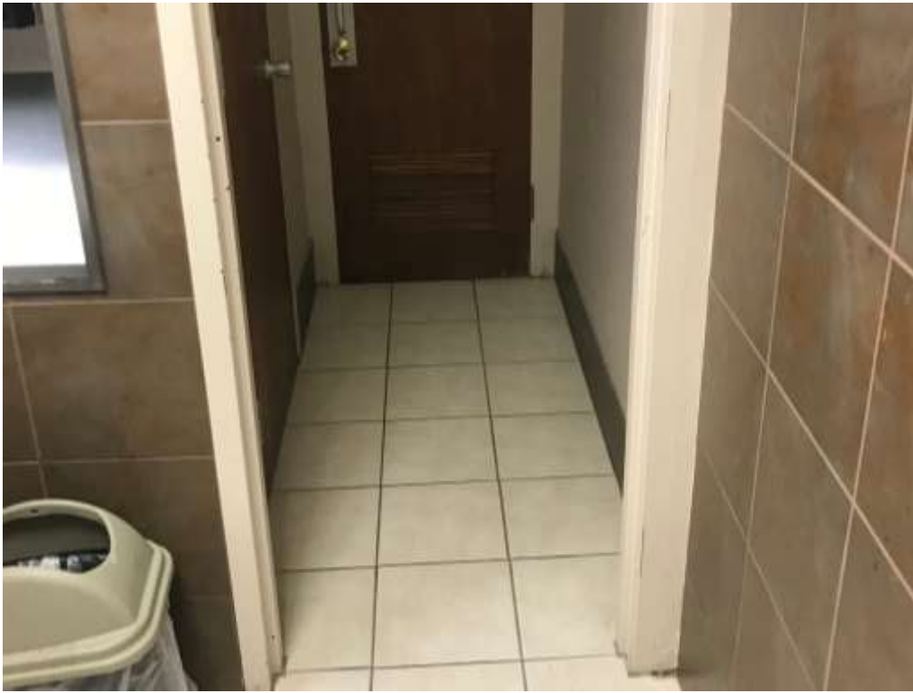
Narrow and inaccessible entry space in restrooms of 8420 Building
