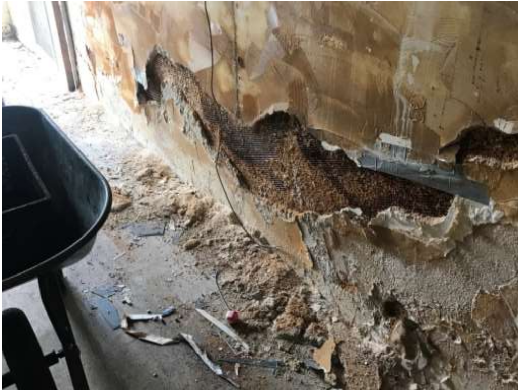
Deteriorated walls and flooring on lower level of former restaurant space of 8420 Building
