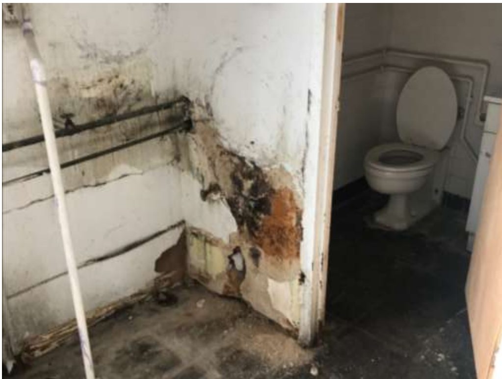
Presence of mold or mildew in former restaurant space of 8420 Building
