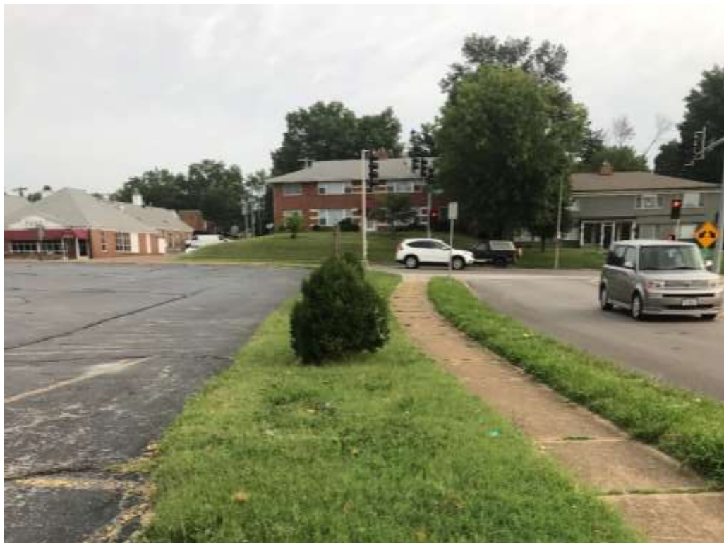
Deteriorated parking surface and sidewalk
