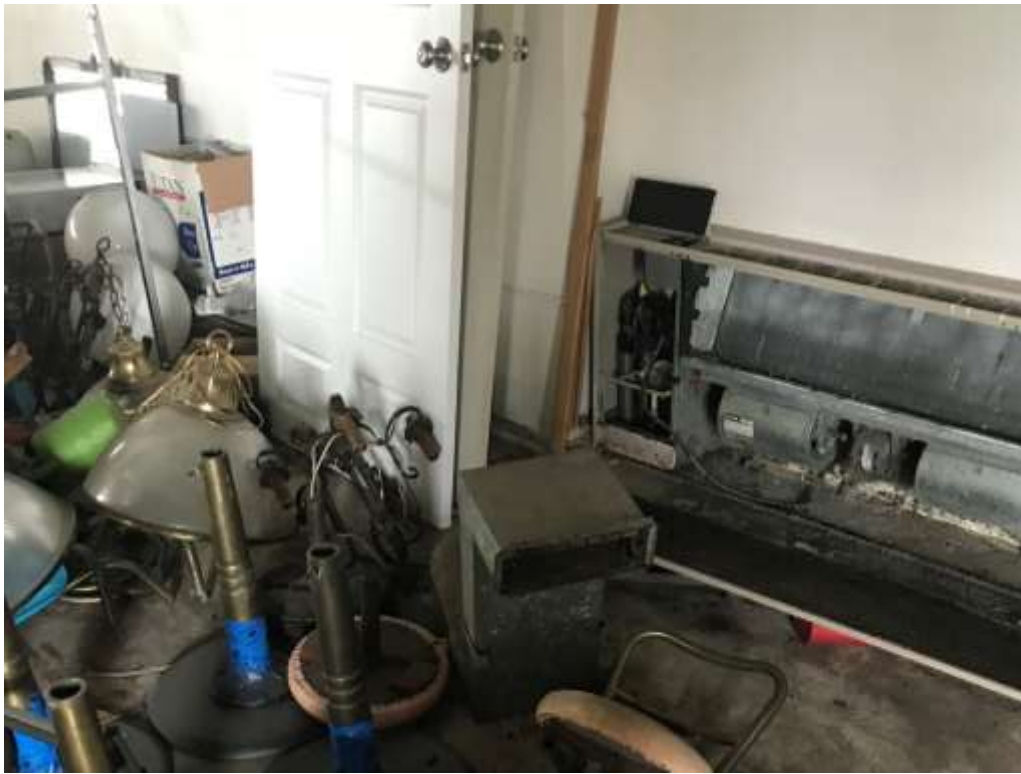
Accumulated materials in vacant retail space of 8420 Building
