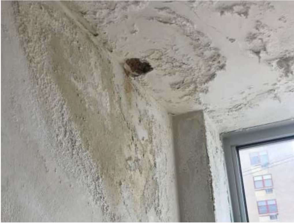
Water penetration lower level entry of 8420 Building
