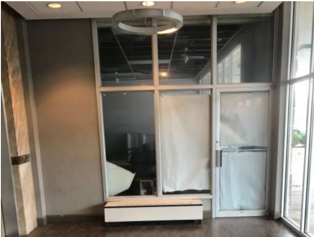
Poor impression of vacant space from 8420 Building lobby entrance
