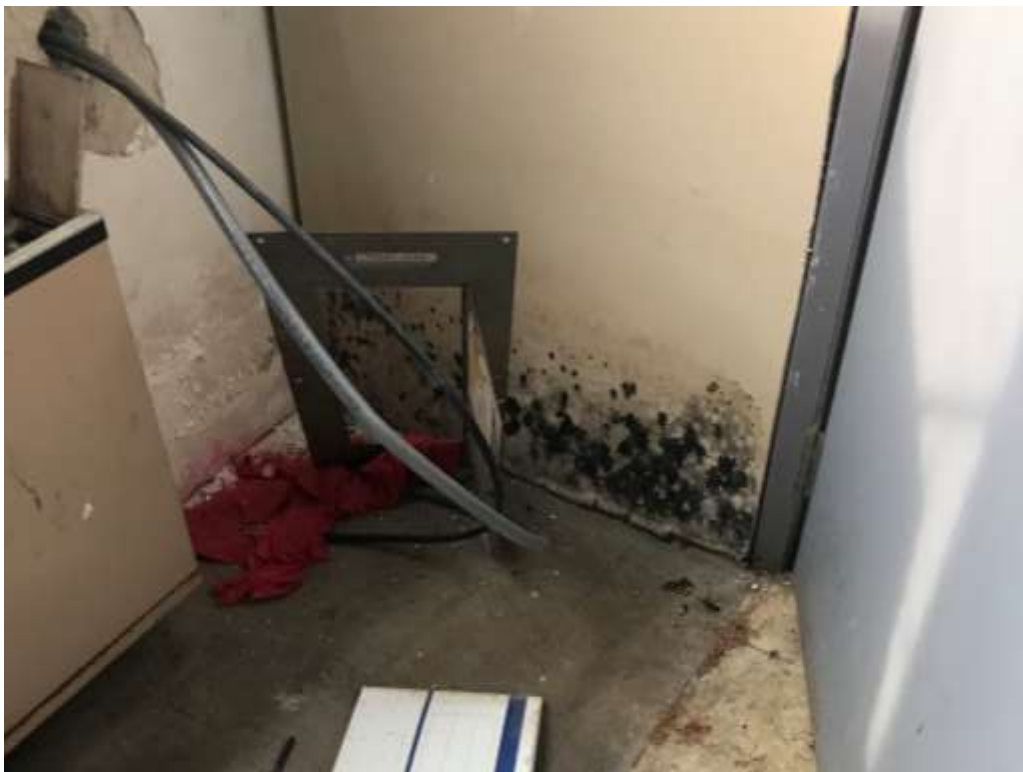
Evidence of mold or mildew in former restaurant space of 8420 Building
