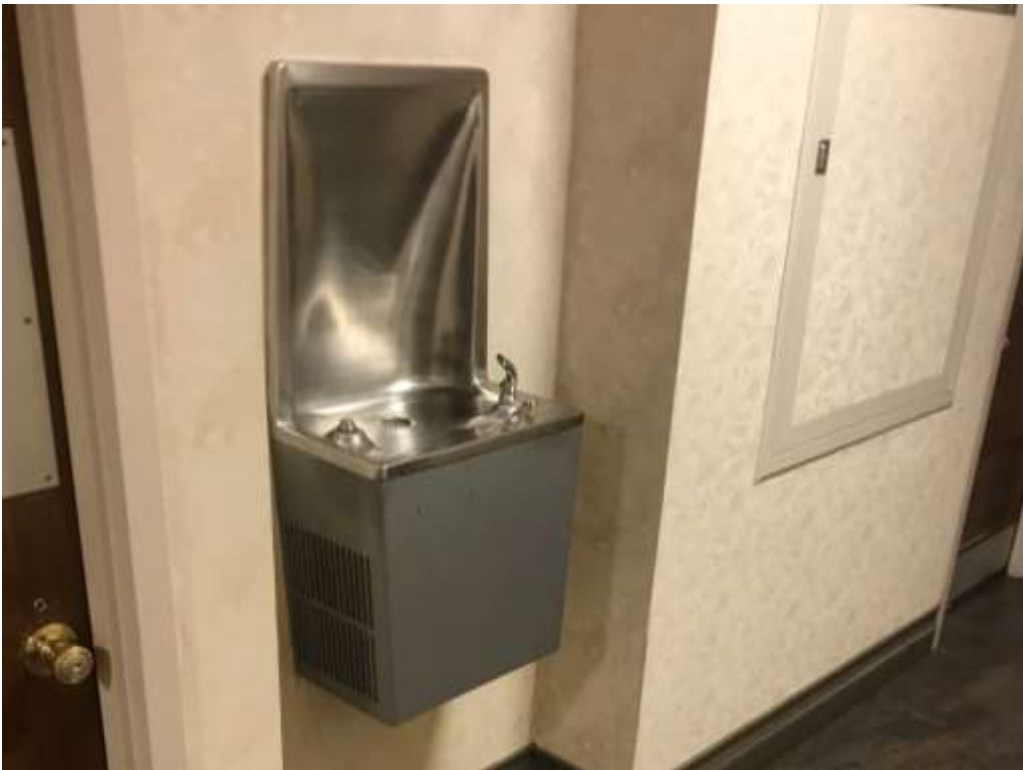
Inaccessible drinking fountain
