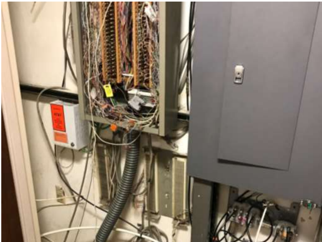
Exposed wiring and panels to public hallway of 8420 Building
