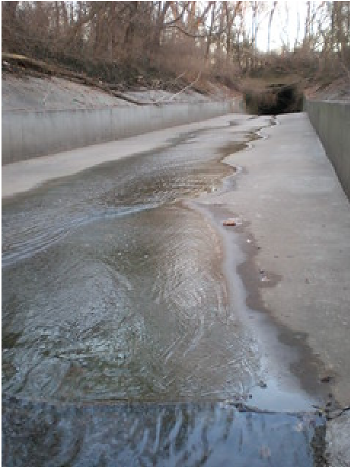
River Des Peres at the entrance to the Tubes (downstream end of study area)
