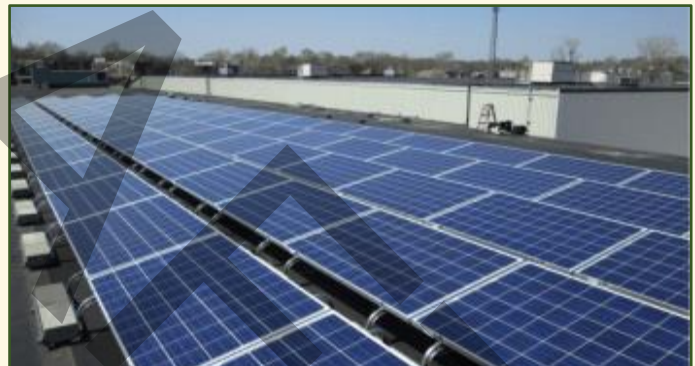
Solar Array found at Washington University in St. Louis
