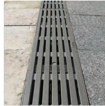
Trench Drains (cast iron)
