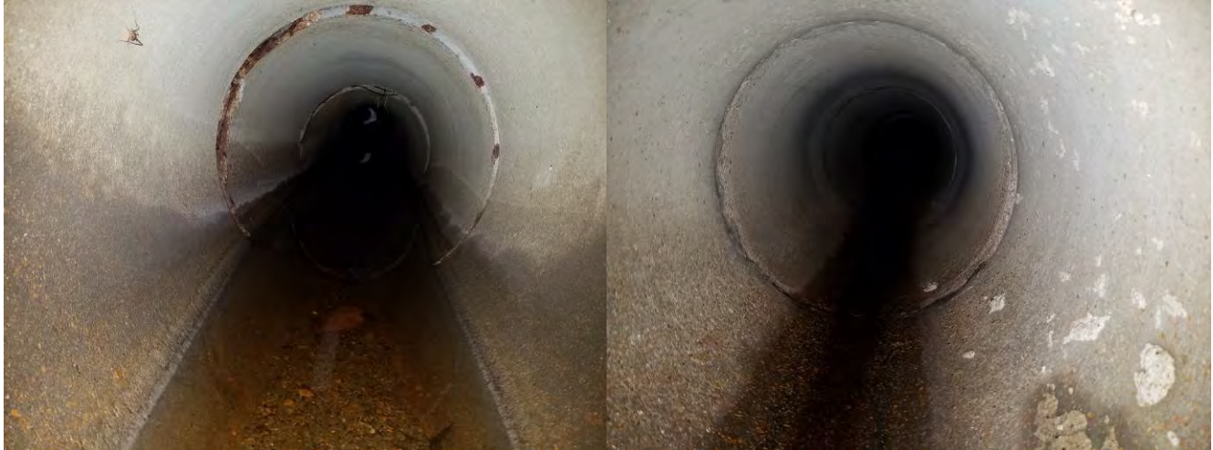
Left Photo: Pipe between structures 17K4-110D & 17K4-044D, taken from 044D looking upstream.
