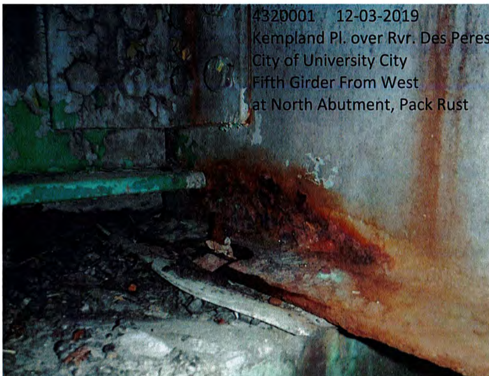
4320001 12-03-2019 Kempland Pl. over Rvr. Des Peres City of University City North Intermediate Box
