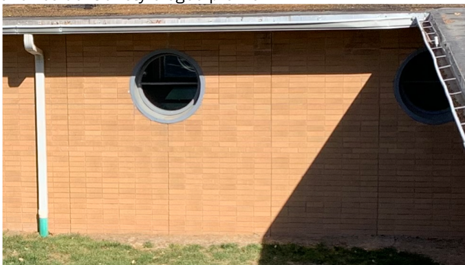
(Existing Courtyard Gutter and Downspout to be replaced)
