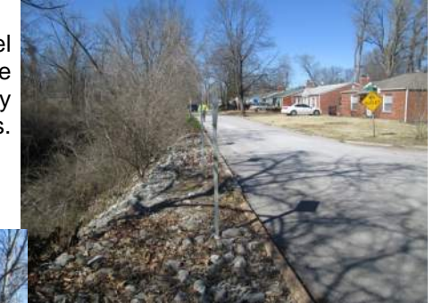
Over-steepened channel banks, and the remains of riprap placed by MSD that has since eroded and slid off the bank.
