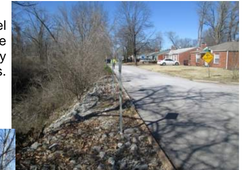
Over-steepened channel banks, and the remains of riprap placed by MSD that has since eroded and slid off the bank.
