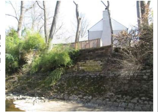
Wood tie wall and WPA block wall. 7425 Shaftesbury Ave is the house behind the wall in the photo.
