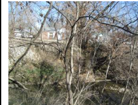
Channel bottom contains riprap, some of which slid off the bank from a previously installed MSD project.
