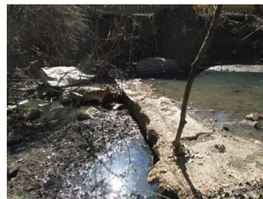
Concrete-encased private sanitary sewer lateral at 7587 Amherst is exposed and possibly leaking. The stream profile drops 2 feet across the lateral.
