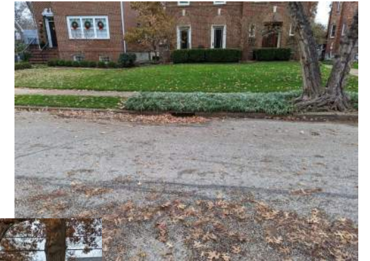
Looking towards the grated curb inlet with side intake between #416 and 414. The side intake is rather narrow and the grate is clogged with leaves.
