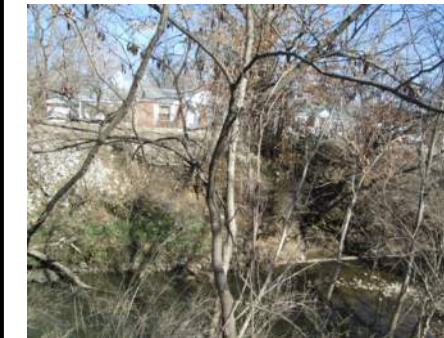
Channel bottom contains riprap, some of which slid off the bank from a previously installed MSD project.
