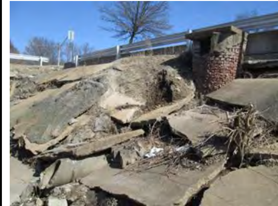
Exposed foundation of the adjacent parking lot.
