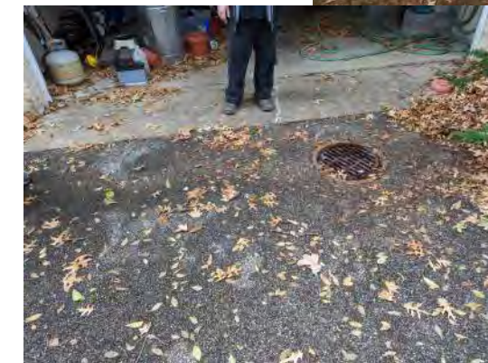
Looking at the ground in front of the driveway at 8436 Old Bonhomme Rd.
