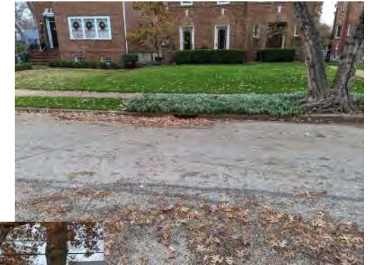
Looking towards the grated curb inlet with side intake between #416 and 414. The side intake is rather narrow and the grate is clogged with leaves.
