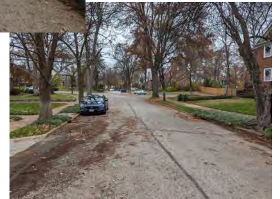
Looking north towards the northern two inlets on W Point Ct. Both are grated inlets with side intakes.
