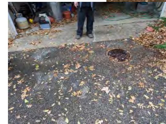
Looking at the ground in front of the driveway at 8436 Old Bonhomme Rd.
