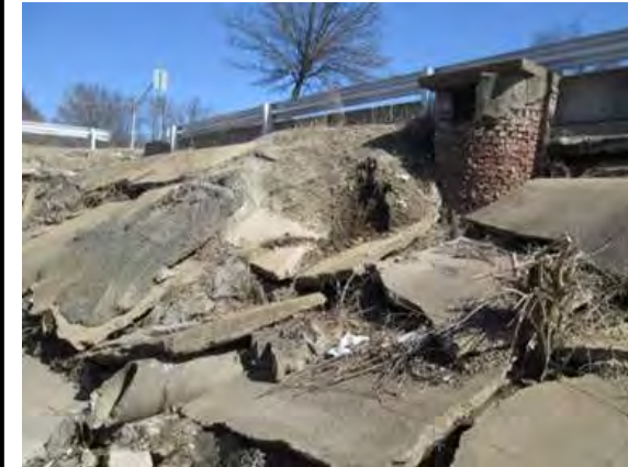
Exposed foundation of the adjacent parking lot.
