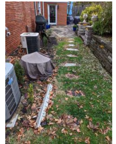
Looking east along the back of 7924 Lafon Pl. A yard drain was installed in an attempt to reduce ponding near the house.
