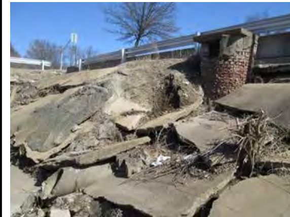
Exposed foundation of the adjacent parking lot.
