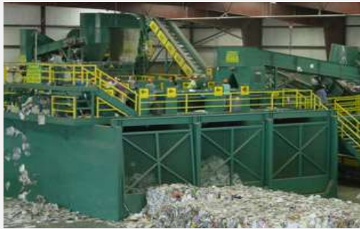
Material Recovery Facility (MRF)
